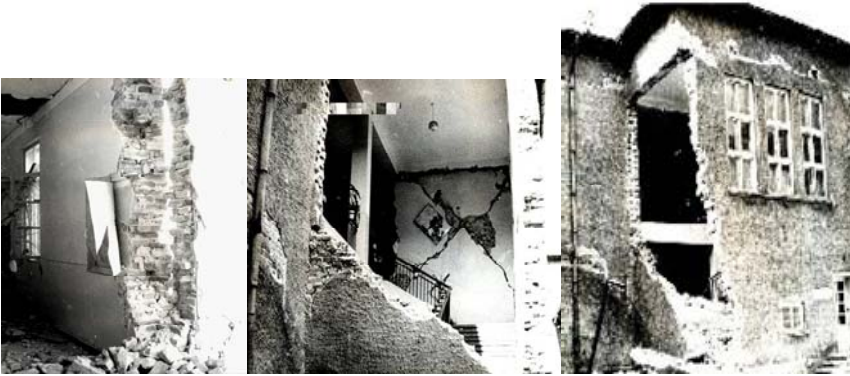
Figure 5: The School in Dve Mogili (1977) – Absence of Steel-concrete Connections.
