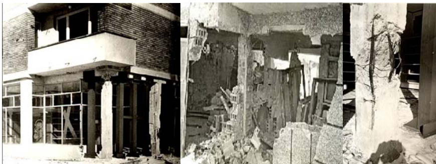
Figure 6: Block of Flats in Strazhitza (1986) – “Flexible” First Floor with Elements of Destructions.
